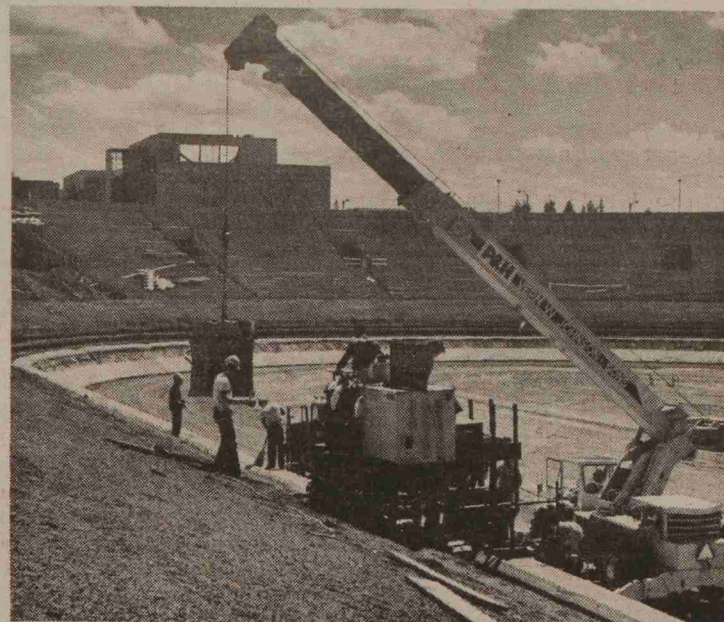
Pouring of slipforms for new seats in Martin Stadium started last week. The stadium is scheduled to be finished Aug. 1. A new track stadium will probably be built on the present Bailey Field and the baseball field will be moved to what was to have been the track site.
